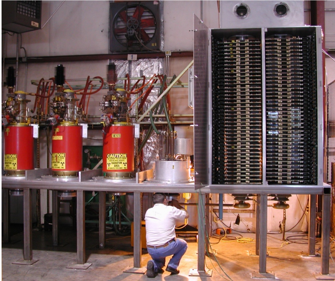
3 turn Secondary with 3 S-band klystrons and a water load installed
